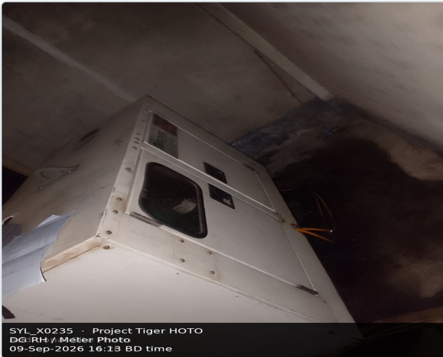
Photo 1 — DG RH / Meter
