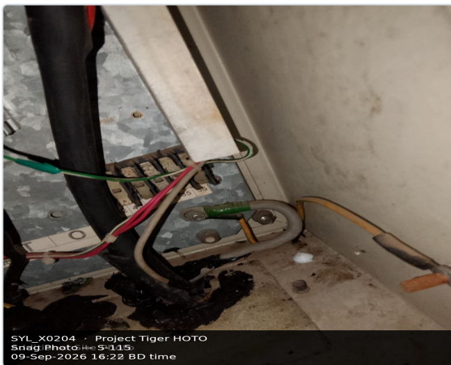
Photo 2 — S-115 — (from HOTO Telegram group photo -- needs review)
