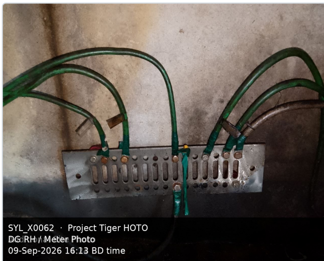
Photo 1 — DG RH / Meter
