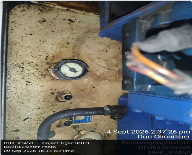
Photo 1 — DG RH / Meter
