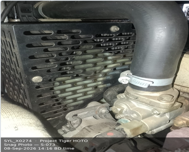
Photo 4 — S-073 — The radiator is full of dust
