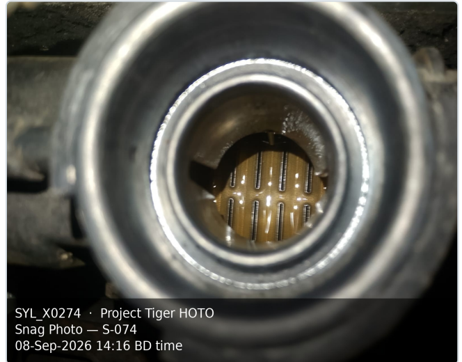
Photo 5 — S-074 — No water in site radiator
