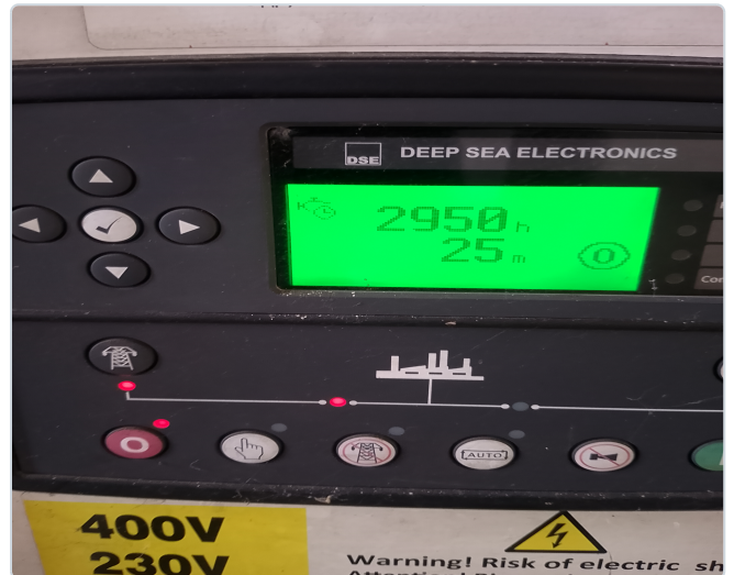
Photo 2 — DG RH / Meter
