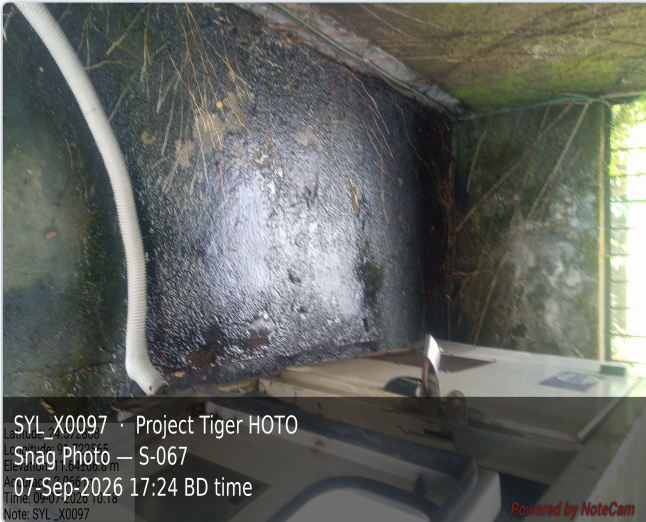
Photo 4 — S-067 — DG room dusty
