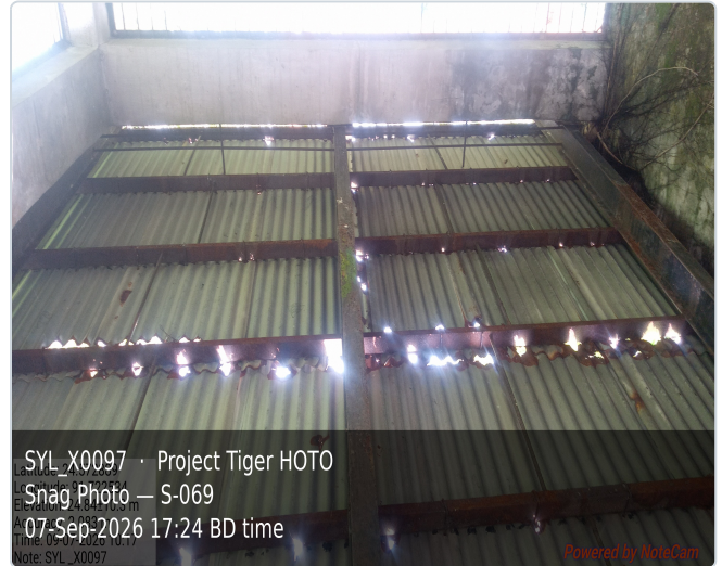
Photo 5 — S-069 — DG room roof tin faulty
