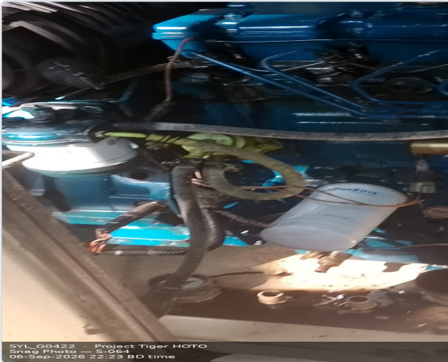
Photo 4 — S-064 — No servicing date found.
