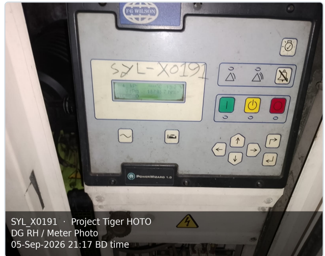
Photo 2 — DG RH / Meter
