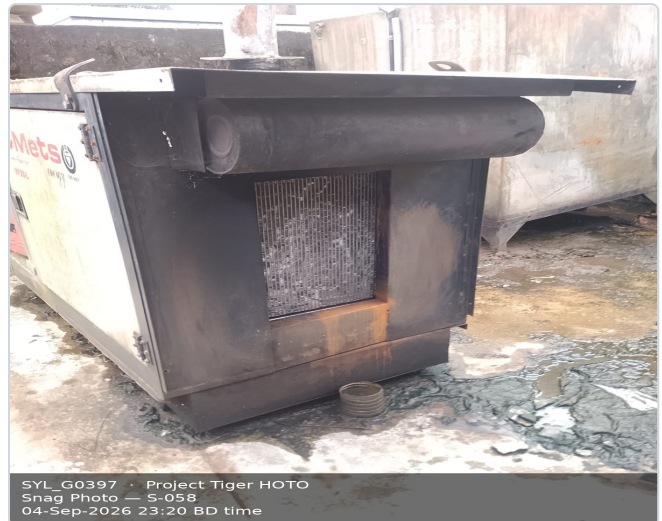
Photo 7 — S-058 — DG back site canopy missing
