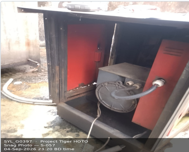
Photo 6 — S-057 — Font site canopy missing
