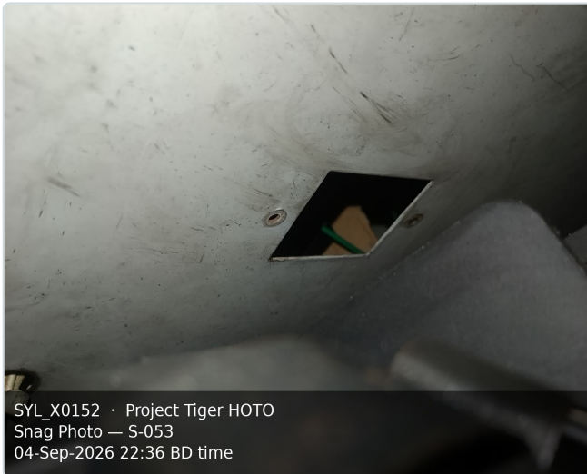
Photo 4 — S-053 — DG power breaker faulty
