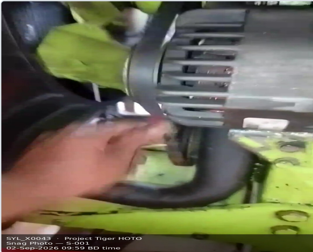
Photo 4 — S-001 — DG Fan Belt Loose
