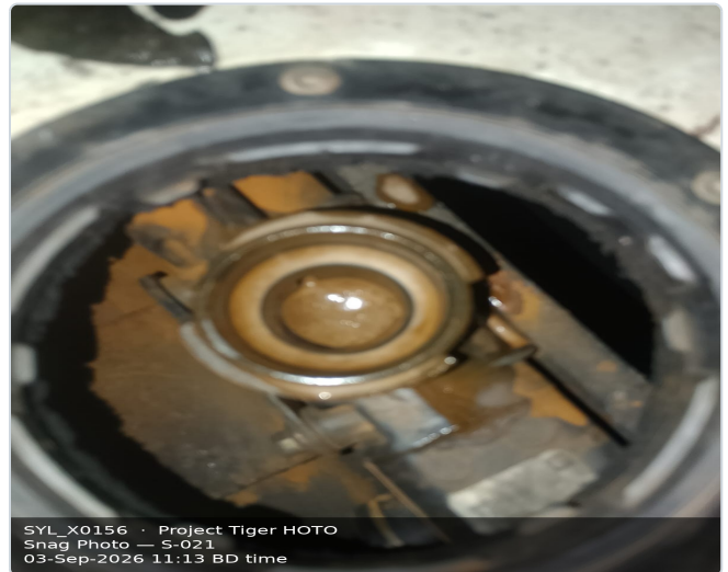
Photo 5 — S-021 — Radiator full block dust
