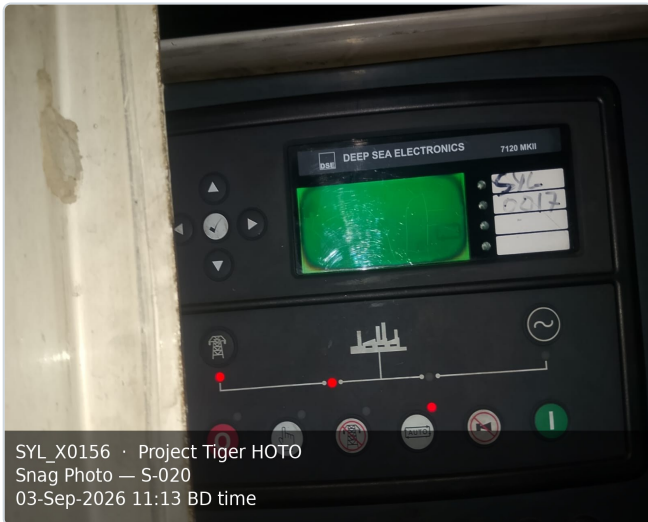
Photo 4 — S-020 — Dg controller display not clean, Nothing on the display is visible
