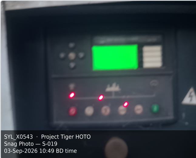
Photo 4 — S-019 — Dg Controller display not visible
