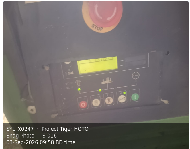
Photo 5 — S-016 — DG controller install proper way
