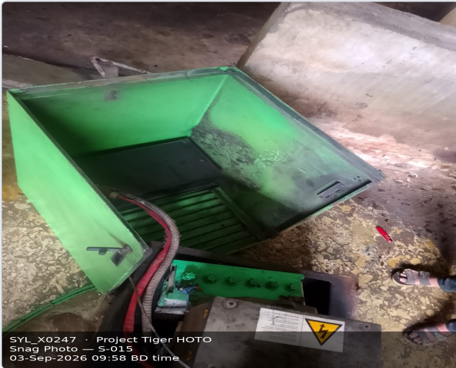
Photo 4 — S-015 — DG canopy broken
