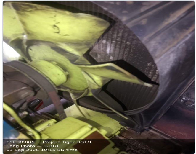
Photo 5 — S-018 — Radiator s blocked with dust.
