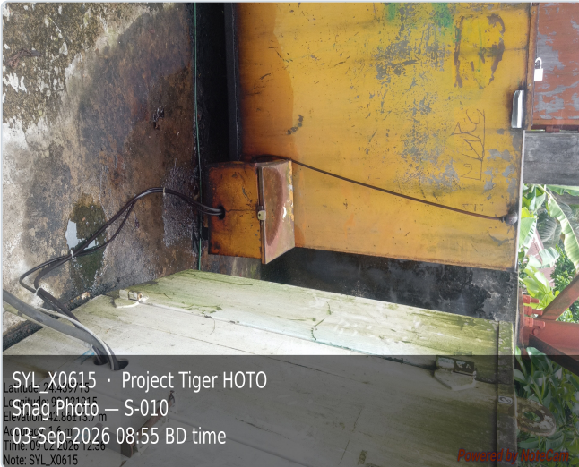
Photo 4 — S-010 — Fuel Pipe ( )
